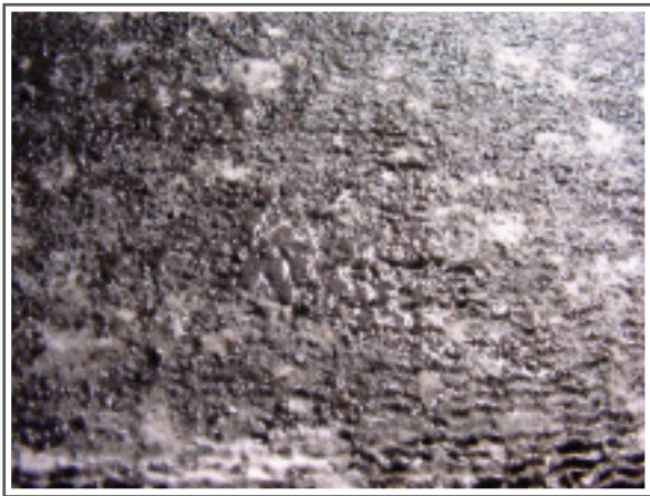
Cooling Coil completely blocked with fungal "cocktail". Negligable air was able to pass through this coil.
