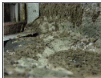
<< Mould growing on internal insulation
