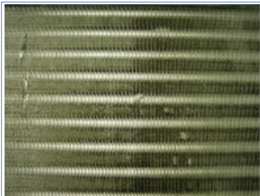
The same coil after Decontamination
